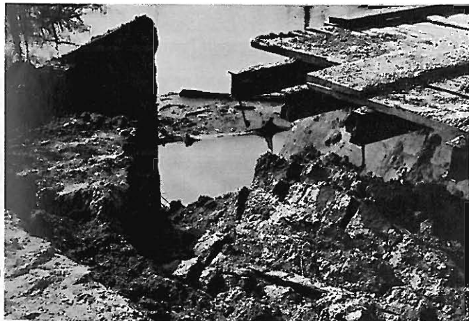
This large gap between the bridge end and roadway was created when a concrete header fell over on the State Highway 13 bridge near Humphrey
