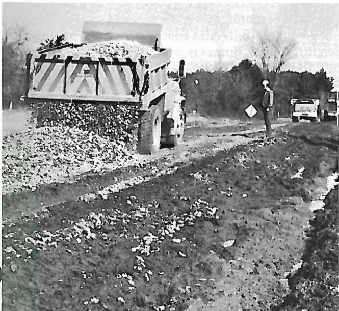
Nearly 600 cubic yards of rock and gravel were dumped on S.H. 321 in an effort to repair the road after it thawed and turned to mud.
