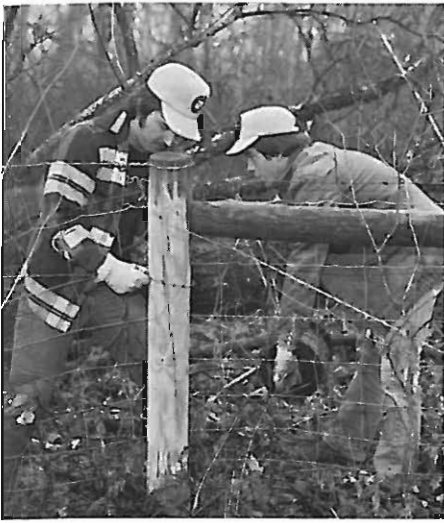
Randy Rearden, left, 2 years service, and Mike McBride, 1 year service, repair fence along Interstate right of way.
