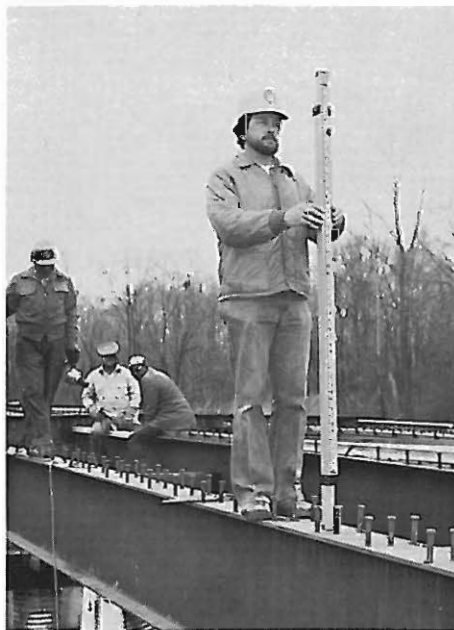
Larry Myers, Construction Instrumentman with 16 years of service, checks camber in bridge "I" beam.
